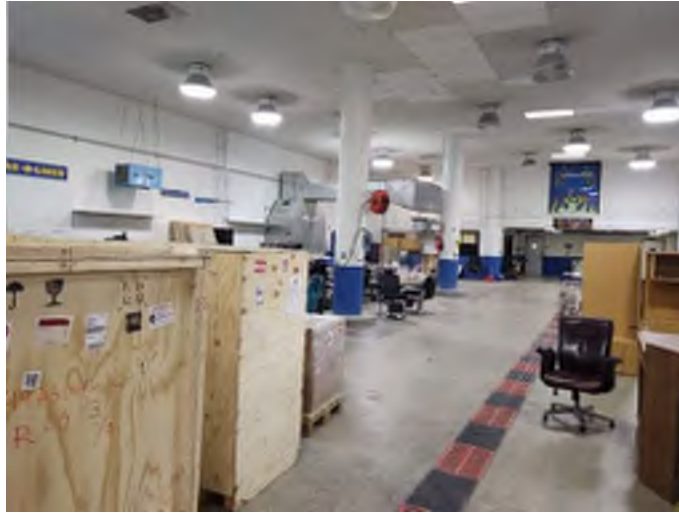
Figure 13 RFC Low Bay Metal Halide Light fixtures in the East area of RFC
