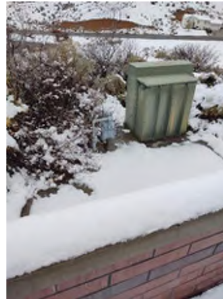
Figure 3 Business Technology Center Pad Mounted 150kVA MV Transformer
